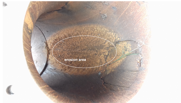
Figure 1. Erosion failure of pulverizer pipe
